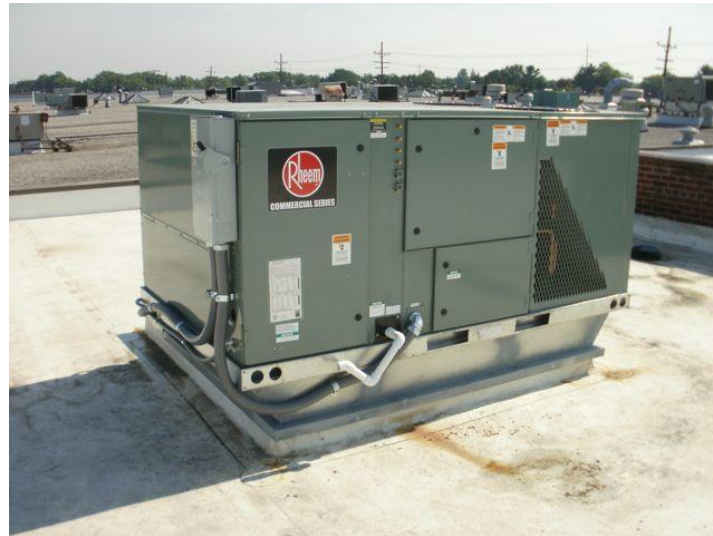
Figure 22 - rooftop air-conditioning unit
